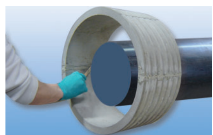
Distribute filler evenly so that the inner surface forms a homogeneous seal surface, smooth with emery cloth, if necessary.
